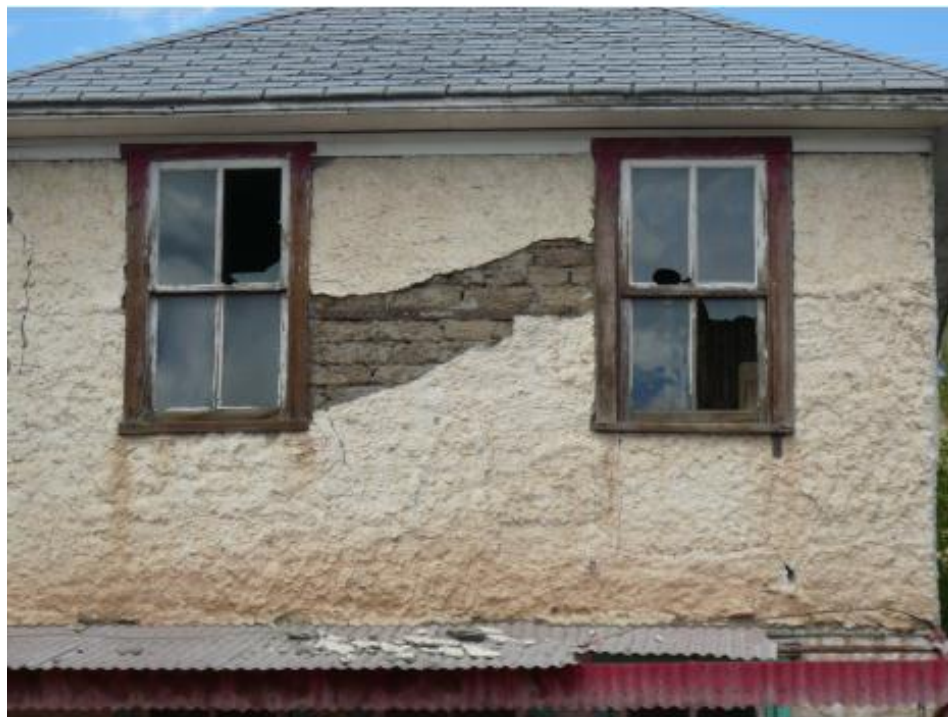
Figure 10-1. Photo of Earthquake Damage from the August 22, 2011 event.
